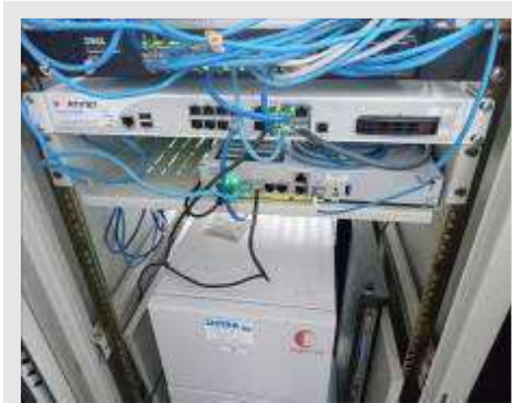
GATEWAY MARCA FORTINET MOD FORTIGATE 200B | Item: 466 |
